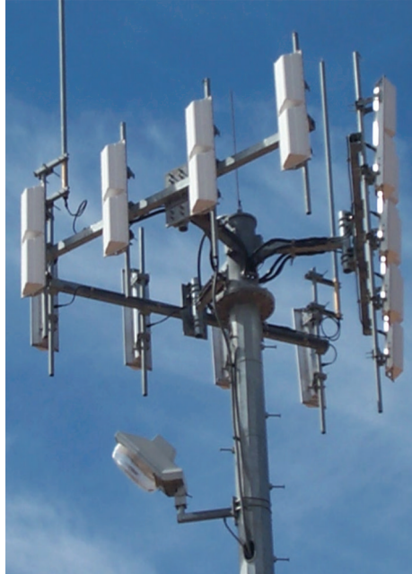
Figure 16.5 Sectorized base-station antenna.
